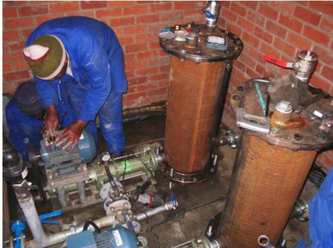
Modifications to Inappropriate Sewer Pump Station Equipment
