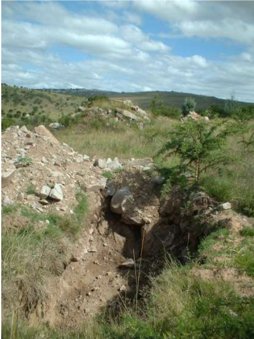
Poor Backfill of Small Bore Sewer Pipe
