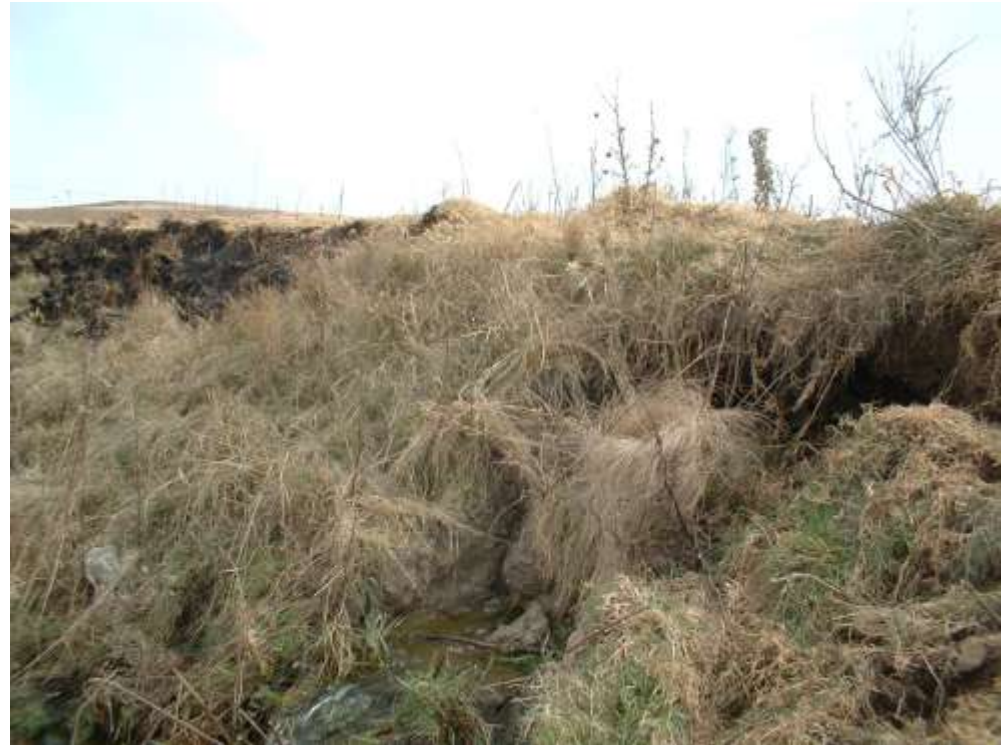
Collapsed Oxidation Pond Wall (Inadequate Design and Construction)
